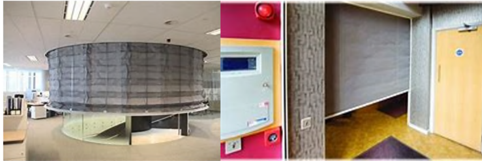
Figure 3: Automatic Fire Barriers
